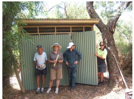
Allan Lim Joon, Pam Bannister, Phil Birchall and Chrissie Dempsey with assembled roo enclosure on site.
