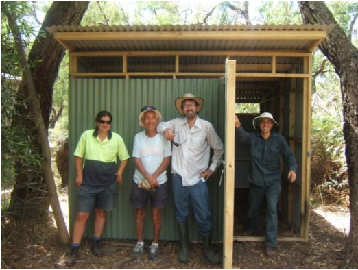
Chrissie Dempsey, Allan Lim Joon, Peter Cooper and Phil Birchall with assembled roo enclosure on site.
